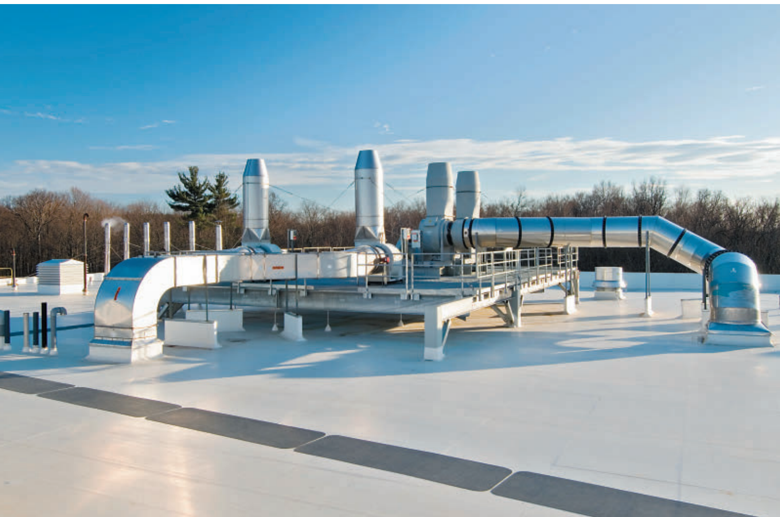
Documenting the condition and functioning of the building envelope, including the roof, and building systems including ventilation, are key when developing a Comprehensive Energy Management Plan.
