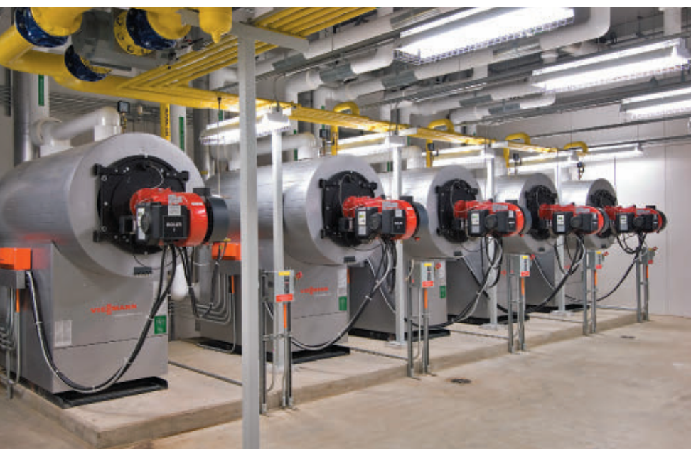
Boilers and other components of a lab's HVAC system, as obvious elements of a building's energy system, require consistent attention and maintenance as part of a Comprehensive Energy Management Plan.
