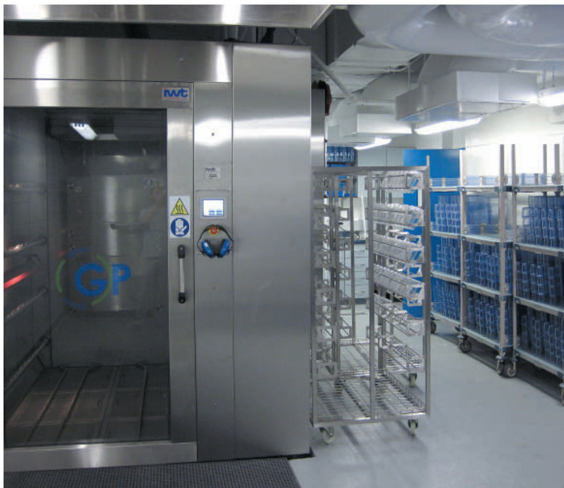
Large, dedicated cage-wash areas, with exposed ceilings, substantial floor drainage and ample space for storage of clean tanks. Image: Erik Sanders
